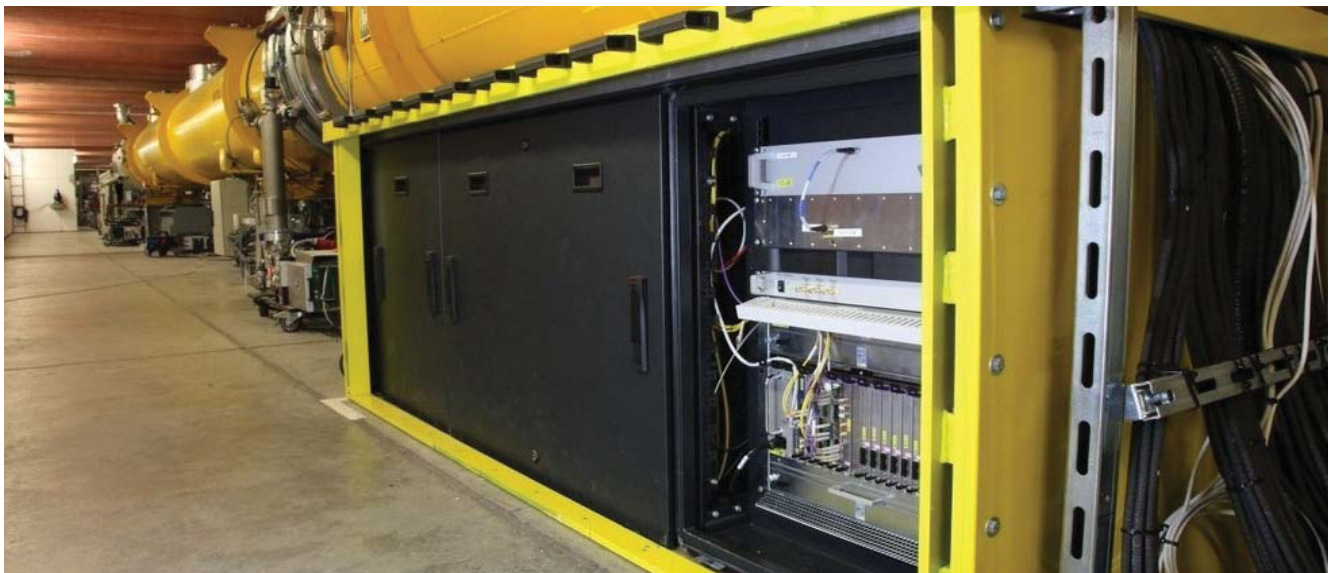
Fig.: Fully functional timing/LLRF control system based on MTCA.4 installed in FLASH (Free electron Laser in Hamburg). Generation of ultra-short laser pulses (4.1 nm).
